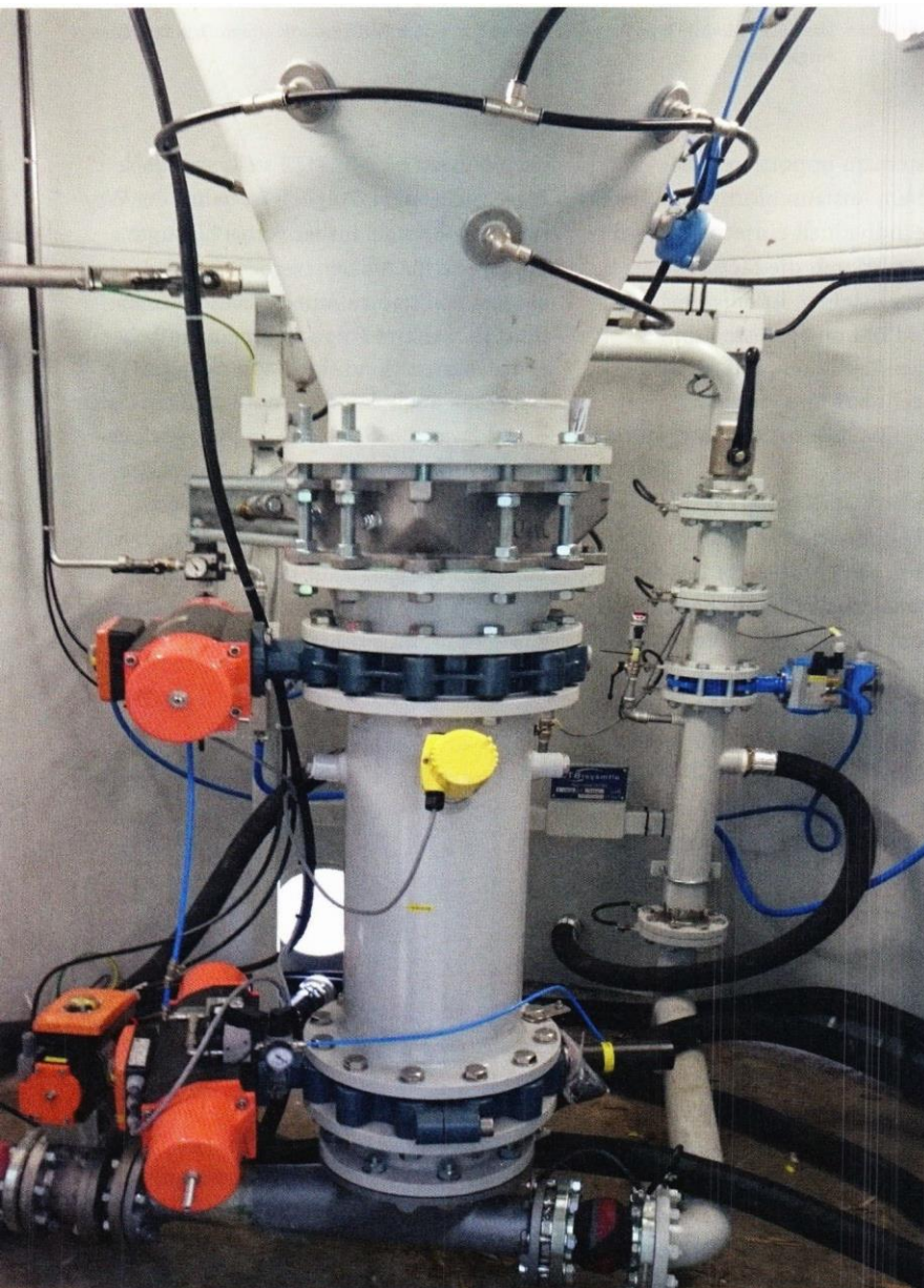
Fig 1: Explosion-decoupling cycle lock doses powder into the feed pipe
